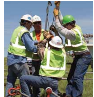
(From left) Jon Sherwood, Jay Ritter, Shane Homan and Paul Taylor secure the conductor so repairs can begin.
