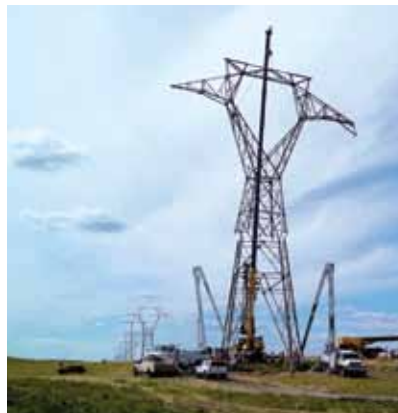
TSM crews assemble the towers in sections and lift them into place.
