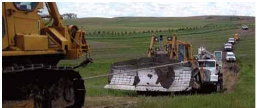
Overcoming the muddy terrain took some slick thinking by TSM crews. They used two bulldozers and a skid plate to pull equipment like this digger derrick truck into place.
