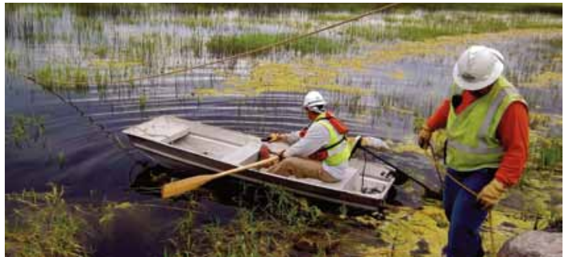
Paul Taylor (in boat) and Vince Smith work to pull a rope across a 1,200-foot wide body of water. The rope is used to pull strawline between two towers on either side of the water. Strawline is cable used to help string and tension conductor.
